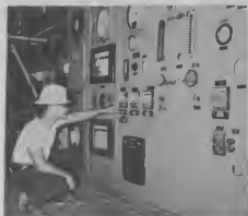
OPERATOR EVARISTO Pinedo checks pitch controller on fire control panel in Powerhouse No. 1.
